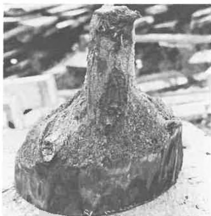
Fig. 13 Spruce pile attacked by limnoria on the exterior and by teredo on the interior. The portion attacked was above the mud line. The portion of pile to full dimension was protected by mud. Here is an example where an eaten pile was salvaged by cutting away the damaged wood and installing a solid timber cap above the re-cut pile.
