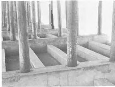
Fig. 15 The lowest point in the concrete is 2' above high water so that the concrete is never immersed in sea water which would otherwise cause spawling due to freezing and thawing. The timber piles are always exposed to complete wetting so that decay will not start due to the combination of creosote and salt preservation.
