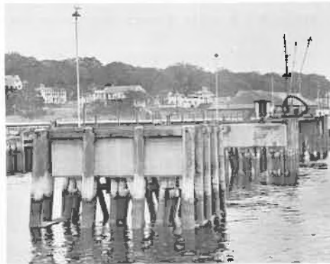
Fig. 16 Tanker wharf consisting of five dolphins at Bucksport, Maine, in the Penobscot River. The low-cost timber piles with the heavy concrete cap provides a stable structure for mooring tankers. The concrete cap shelters the structural piles against rain water decay and at the same time ties all of the battered piles so that they will act together. The mass of the concrete is above highest water so that maximum effective weight will exist for stability. The piles between low water and the concrete were treated with copper naphthanate solution against rotting. These piles are untreated fir since they are in the fresh water of the Penobscot River. This is another example of the advantage of composite construction using timber and concrete.
