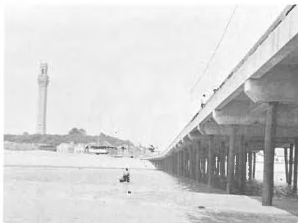
Fig. 14 MacMillan Wharf, Provincetown, Mass. This wharf is a good example of composite construction utilizing creosoted yellow pine piles with cast-in-place reinforced concrete caps. The longitudinal stringers were precast to minimize form work over water and to enable rapid assembly of the deck system. Forms were then placed between the stringers for pouring a 6" reinforced concrete slab to tie all of the caps and stringers together.
